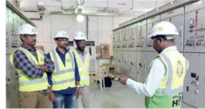
Montaza Substation, Qatar
