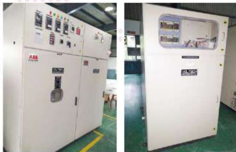
11kV VCB panel & 33kV Metering Panel
