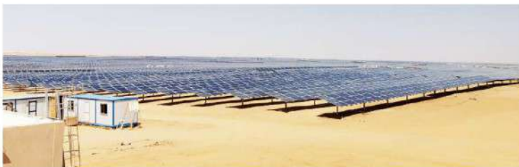
Successfully completed testing & Commissioning work activities for 165.5MW Benban Solar Complex Solar power plant at Benban- Egypt through M/s. Chint (Hong Kong) Co. Ltd.
