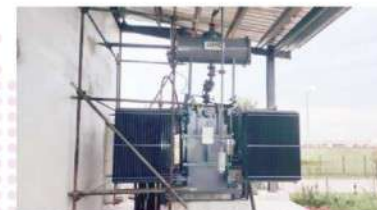
VMC make 3MVA, 33/433v Distribution Transformer - Indorama Ventures PET Nigeria Ltd-Port Harcourt (Nigeria)
