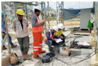
Our Engineers Mr. M. Karthikeyan at PT. RCR Energy Indonesia – 37 MW Combined Cycle Senipah Project at Kalimantan, Indonesia
