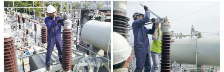
Our Engineers Mr. K. Nesamani, Mr. V. Arun Bernathsa and Mr. P. Salthish at M/s. Toyo Thai Power Myanmar Co. Ltd, Myanmar - Annual Maintenance Servicing of 12MVA Transformers at 120MW TTPMC Power Plant at Ahlone Yangon, Myanmar
