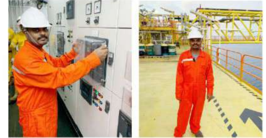
Our Malaysia Country Manager Mr. S. Parthasarathy at M/s. PC Myanmar ( Hong Kong ) Limited, Myanmar - Annual Maintenance Services of 4kV and 0.4kV Switchgear/Switchboard at Petronas Yetagun Onshore and Offshore Platform.
