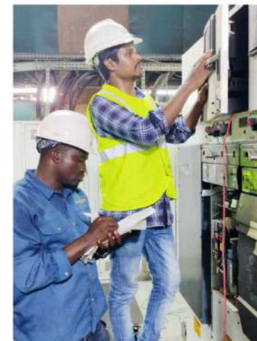
Annual Shutdown Maintenance work for 11kV VCB Panels and Relays at TPUL Sango Ota (Nigeria)
